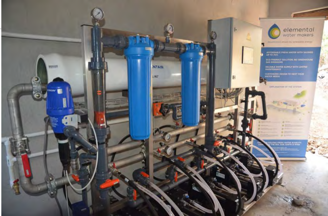
Figure 2 The desalination system of Elemental Water Makers on the BVI
